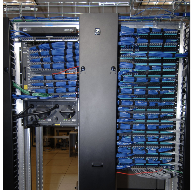
Figure 6: Fellowship's switch and patch panel racks
