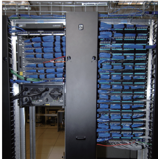
Figure 6: Fellowship's switch and patch panel racks
